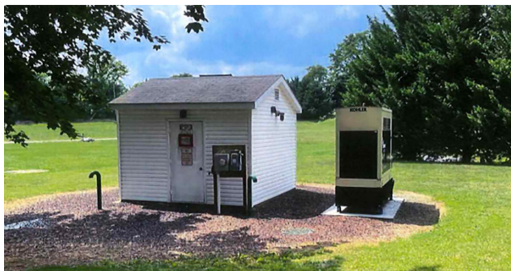
Chip's Meadow Sewer Pump Station
