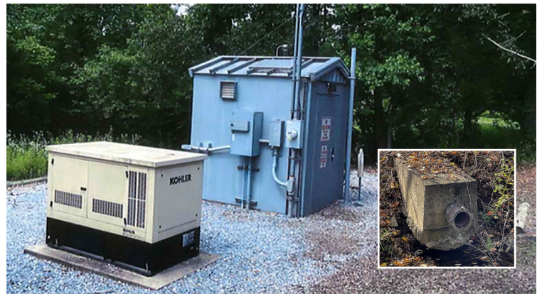
Henrietta Pump Station
